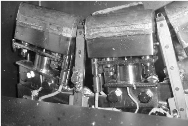
Fig. 4. View of FTU limiters.
